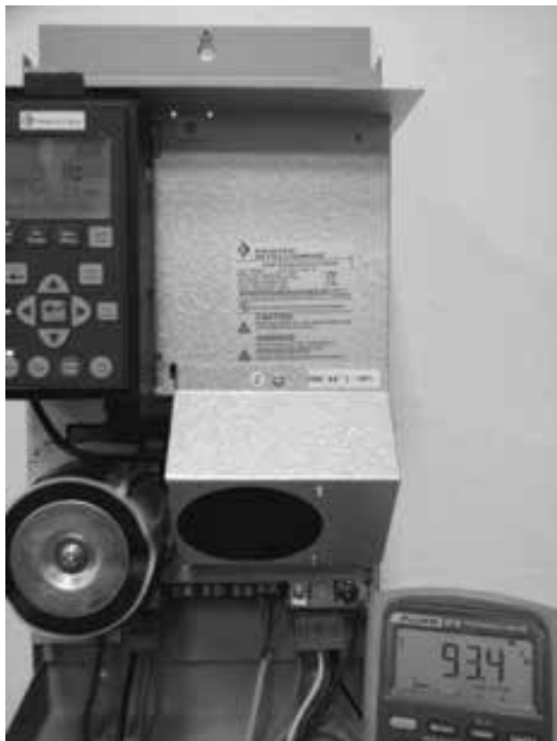
Figure 20. 3 phase 30Hz voltage measurement
