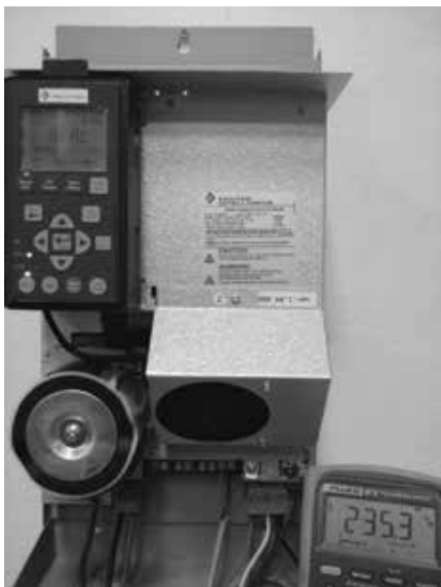
Figure 22. 3 phase 60Hz voltage measurement
